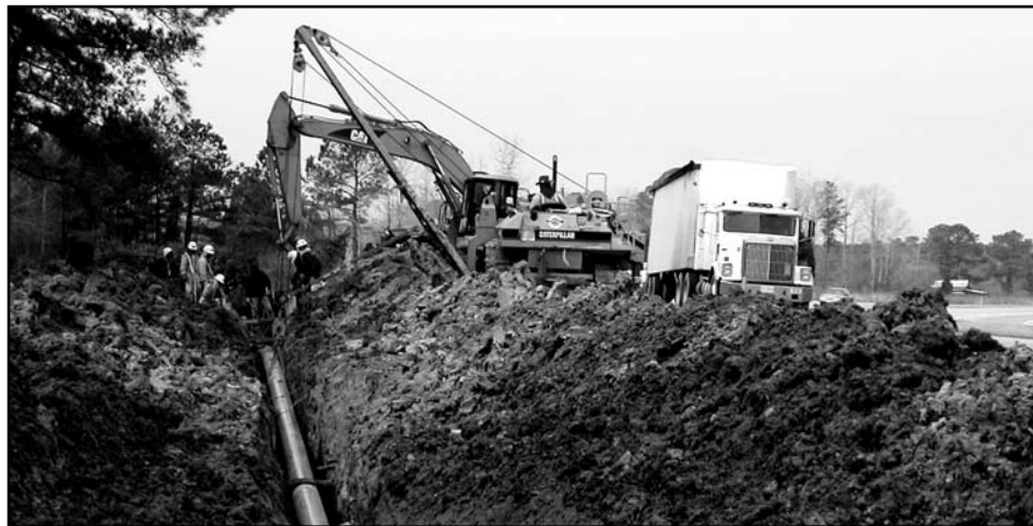
Construction crews work on the ENCNG pipeline in Martin County (CJ photo)
