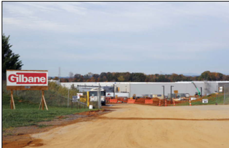
Apple is constructing a second building at its data center in Maiden, N.C. (CJ photo by Don Carrington)
