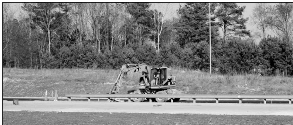
Slow work, such as that shown above on the incompleting I-540 in Raleigh, is common on projects throughout the state. (CJ photo by Don Carrington)
