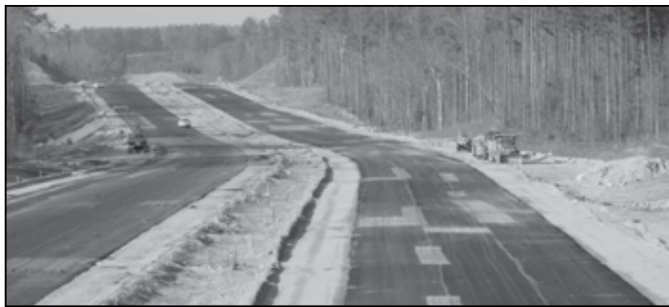
Many more lane miles, like these under construction in Wake County last year, will be needed in North Carolina in the next 25 years. A national study by the Reason Foundation says Greensboro, Wilmington, Gastonia, and Concord face traffic similar to Pittsburgh and Cleveland today. (CJ file photo)
