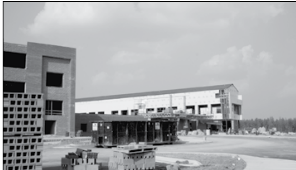
State leaders say a lot more construction like this project at Panther Creek High School in Wake County last fall will be needed in the next five years. (CJ file photo)
